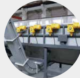
Float-sink Washing Tank
